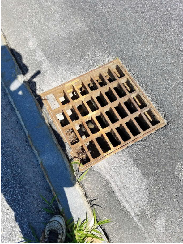
Drop inlet for stormwater from road into wetland.
