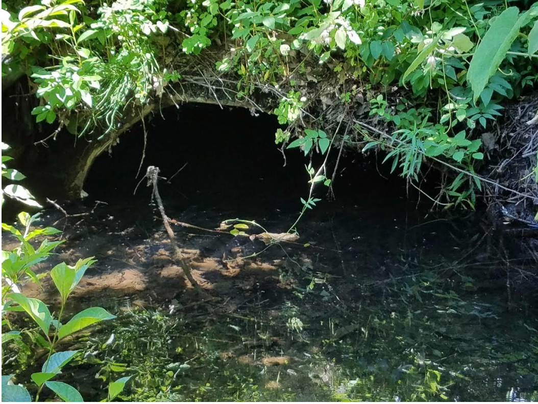
Culvert (6' squash pipe) under Waukegan Road, carrying stream from south side of road into wetland.
